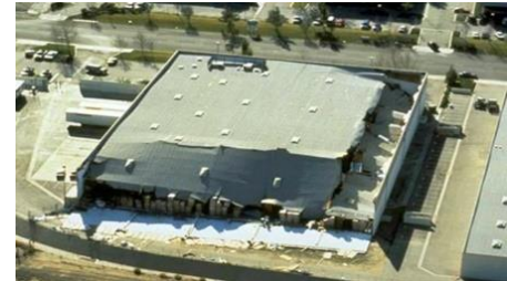
Example of Failure in Concrete Tilt-Up Building
